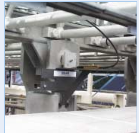
Extensometer as a probe on a steel structure.
