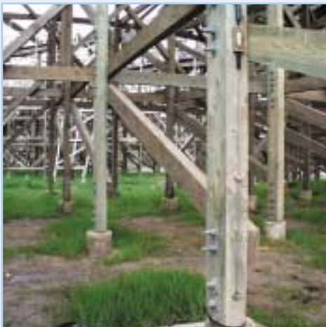
Extensometer on a wooden structure.
