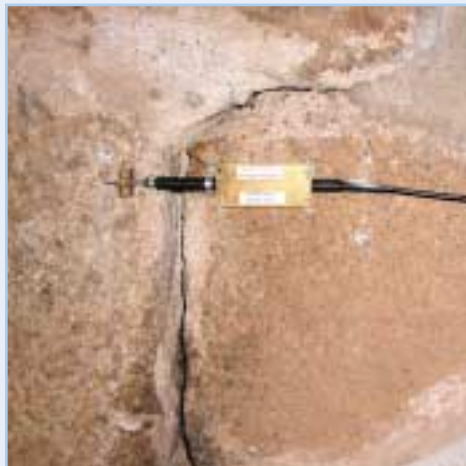
Extensometer as a fissure monitor.
