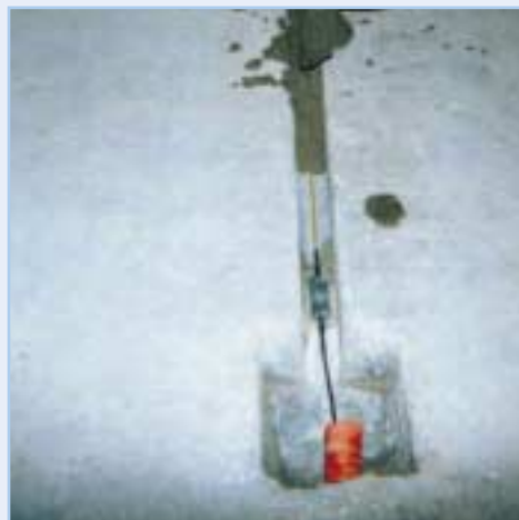
Optical Strand post-installed in mortar.
